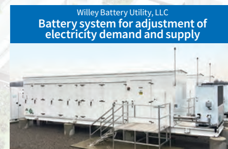
This battery has been adopted for large battery systems for adjustment of electricity demand and supply in the United States.
