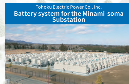
This battery has been adopted for measures to balance the demand and supply due to diffusion of recyclable energy.
