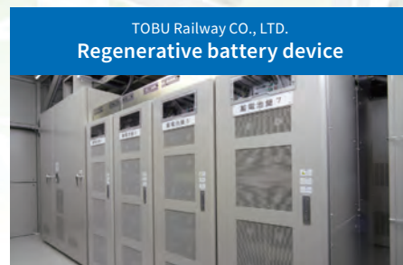
This battery has been adopted for regenerative battery devices to effectively use the regenerative electricity generated by deceleration of a railcar.
