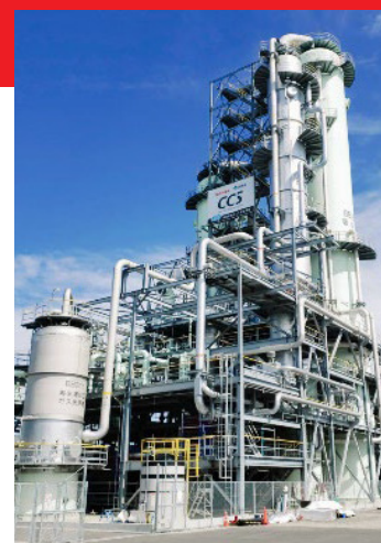
Figure 1. CO 2 Capture Demonstration Plant
