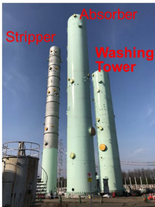
Figure 7. Towers in the Demonstration Plant
