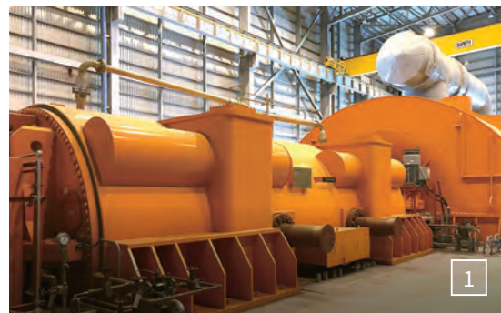
1 Vinh Tan 4 Thermal Power Plant, Vietnam
