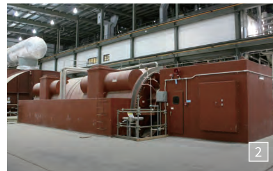
2 Coal Fired Thermal Power Plant, North Carolina, United States
