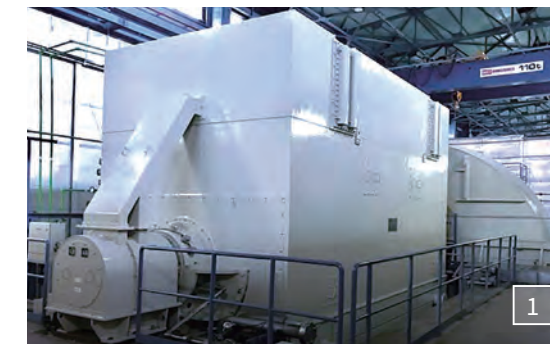
1 Mindanao Coal-Fired Thermal Power Plant, Philippines
