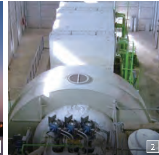
2 Mindanao Coal-Fired Thermal Power Plant, Philippines
