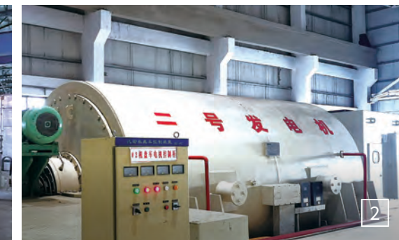
2 Manzhouli Dalaihu Project for 2X200MW Cogeneration Power Plant, China
